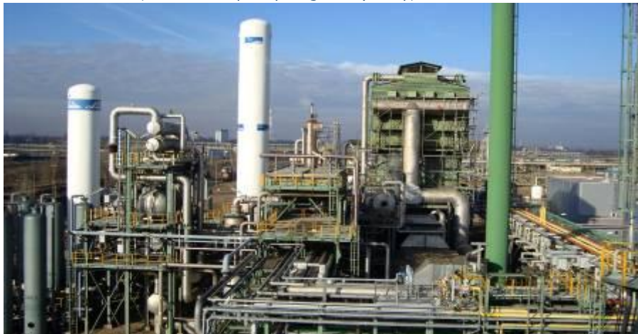
Steamreformer I (35.000 Nm 3 /h hydrogen capacity)
